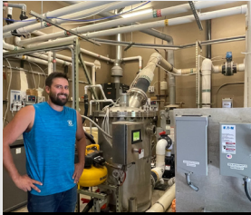
Eli Schlagel of Front Range Recreation shows off the new pump room, with its state-of-the-art technology and systems.
